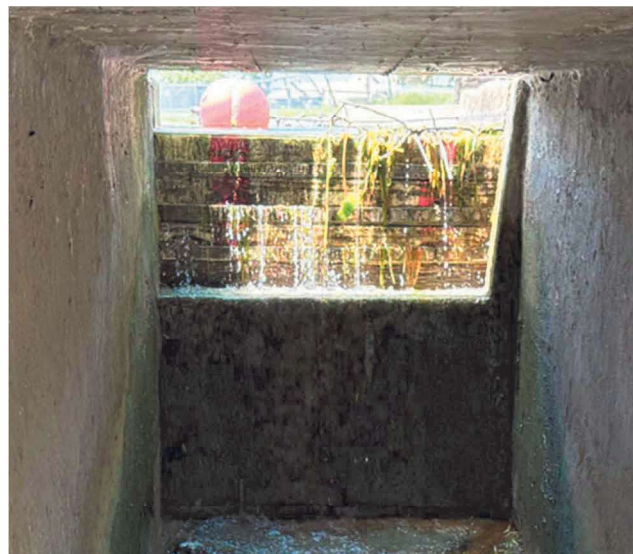
Figure 14 North Channel with (3) Weir Boards
